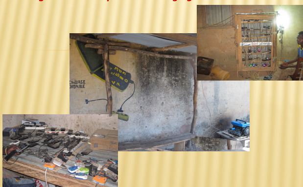
Figure 4. Mobile phones recharging units
